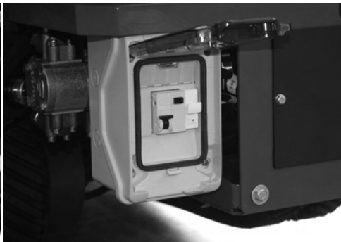
Fig. 144 Main supply switch
